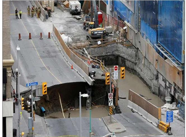
Example: of sink hole on Rideau Street, Ottawa
